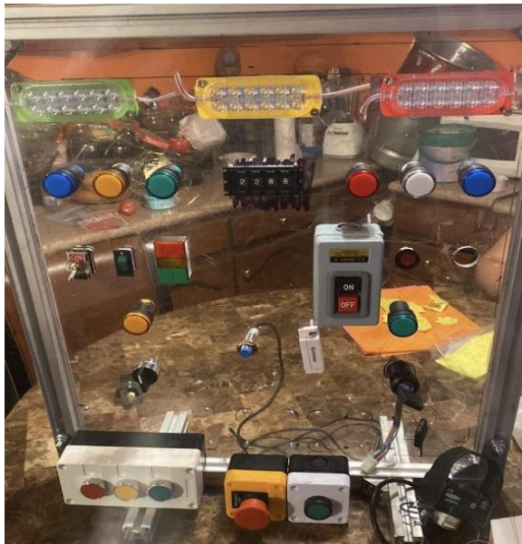
Figure 5. Drives on structure
