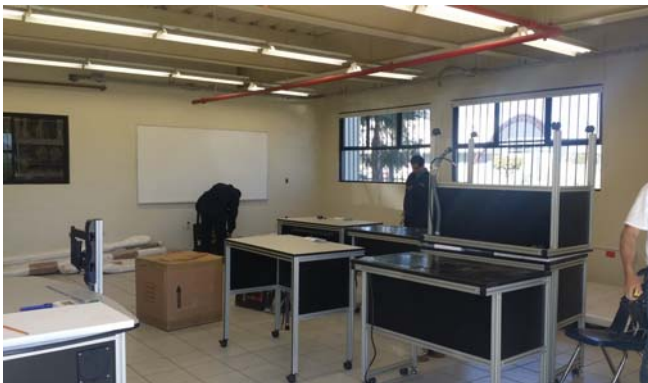
Figure 1.2 Supervision and Installation of equipment, with the security and proper precautions, during a period of 3 days.
