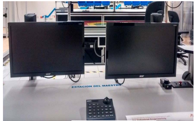
Figure 2.1 Central of monitoring station.
