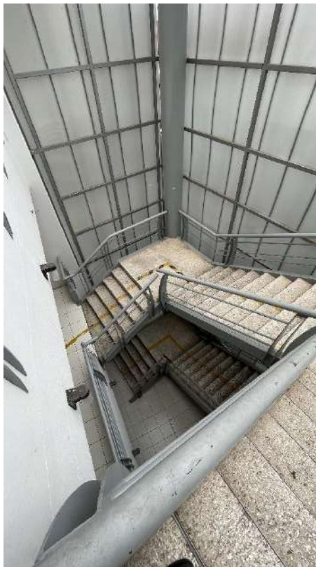
Figure 1. Technical inspection of vertical circulation cores. The audit identified the need for high-visibility anti-slip treatment and reinforcement of handrail ergonomics to comply with local safety standards (NOM-001-STPS).
